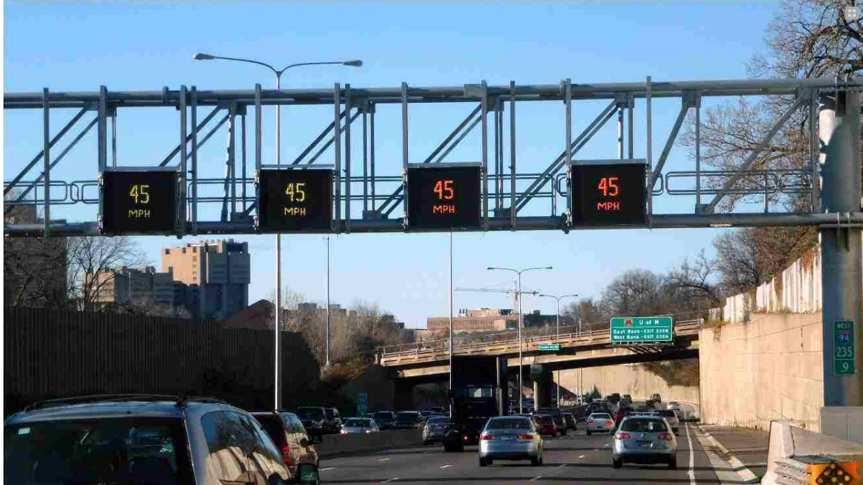
Figure 5. Active Traffic Management system on I-94 (Source: http://ungemah.com/sh_projects/i-94-managed-lanes-study-phase-1/ )
